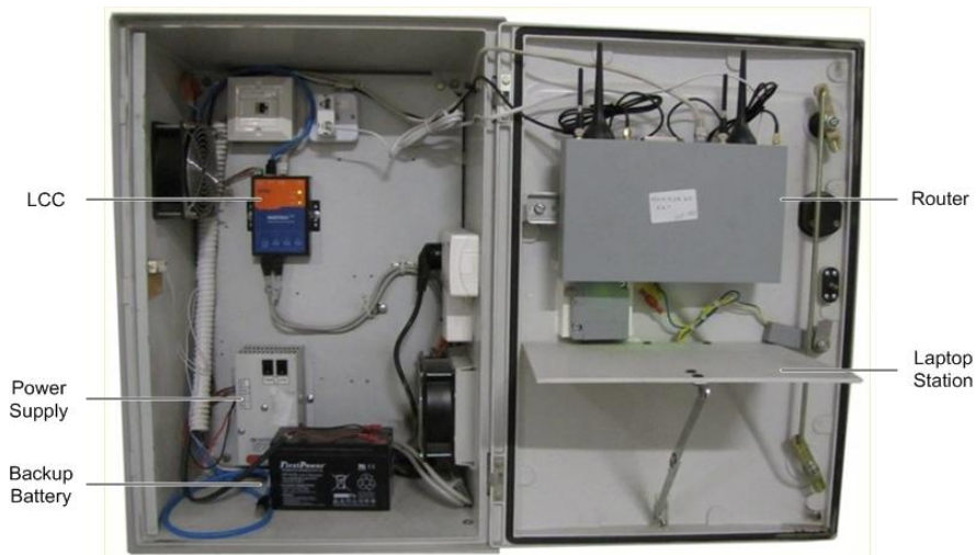
Figure 89: Communication Cabinet Wiring
